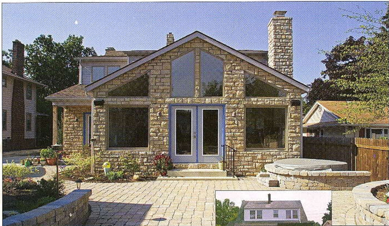
Above: The remodeling plan included demolishing the old kitchen, knocking out the back wall of the house and constructing a new, larger kitchen and dining and entertaining area. Inset: An existing deck was removed and the patio torn up to make way for the addition and a new guest-friendly outdoor area.
